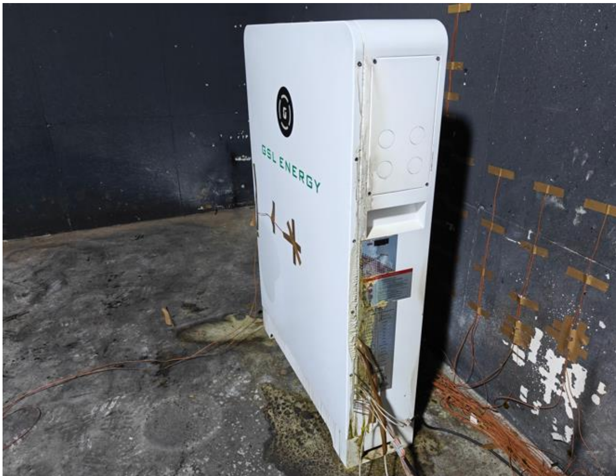
Figure 22. Photo 02 of initiating BESS Unit after test
