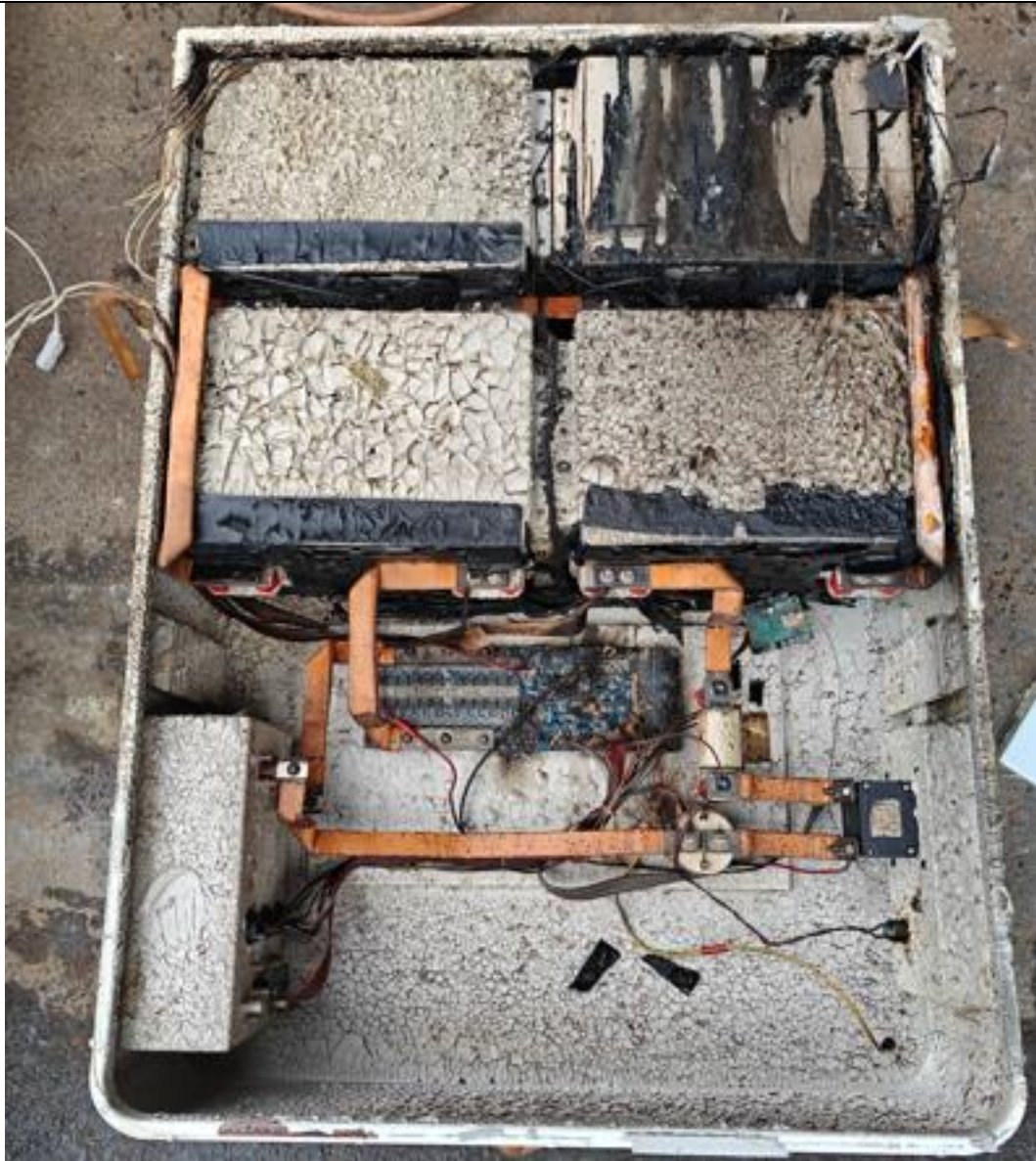
Figure 15. View of location of module that exhibited thermal runaway within the initiating unit
