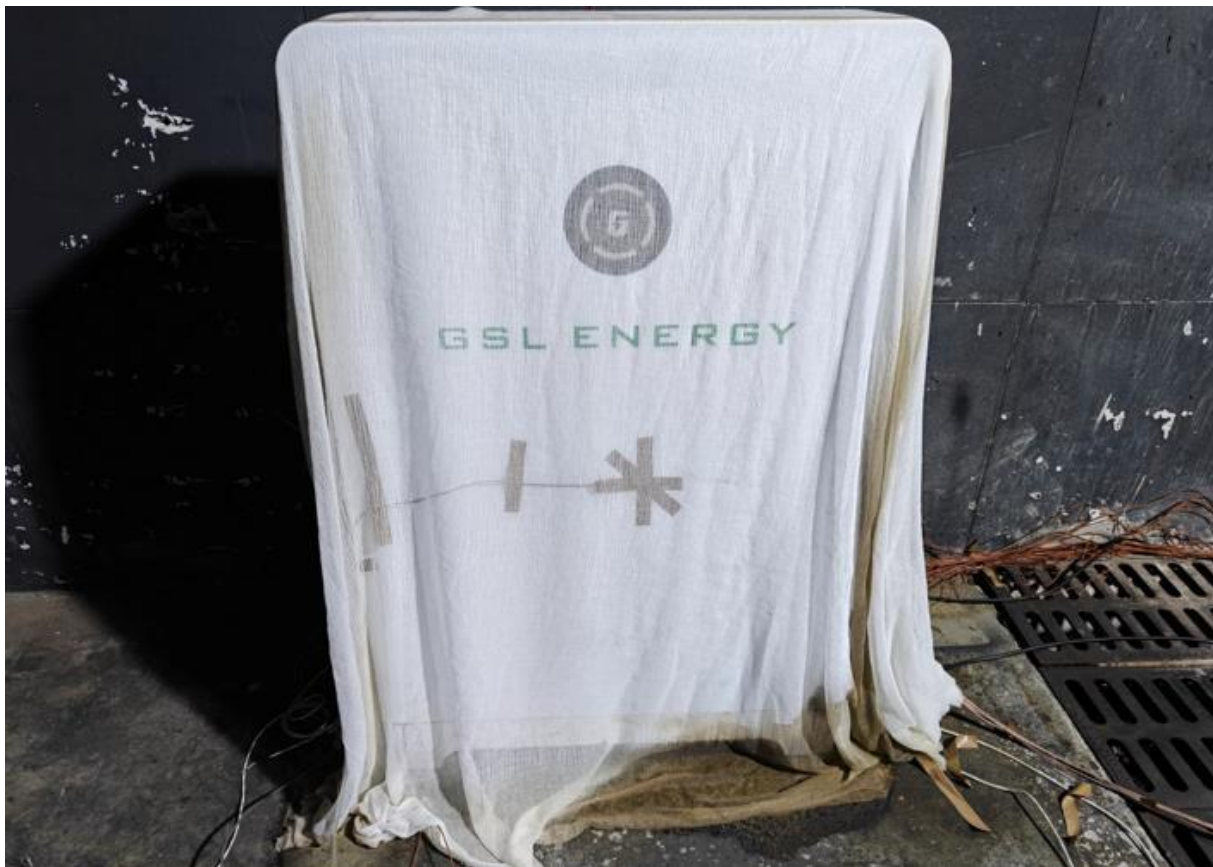
Figure 21. Photo 01 of initiating BESS Unit after test
