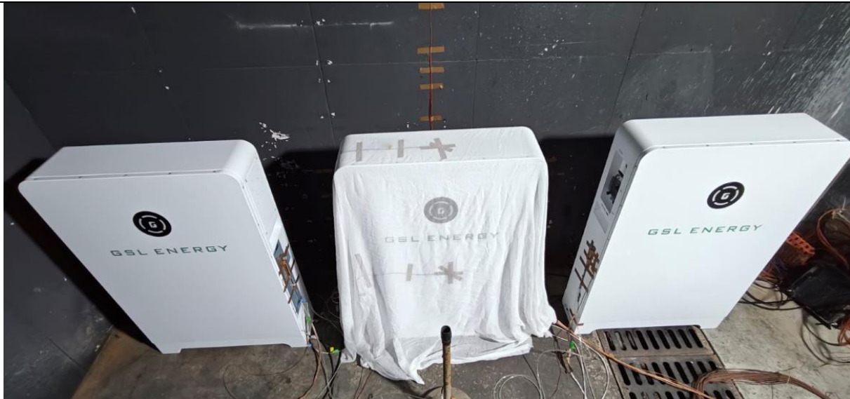
Figure 10. View of positioning of BESS units in testing room.
