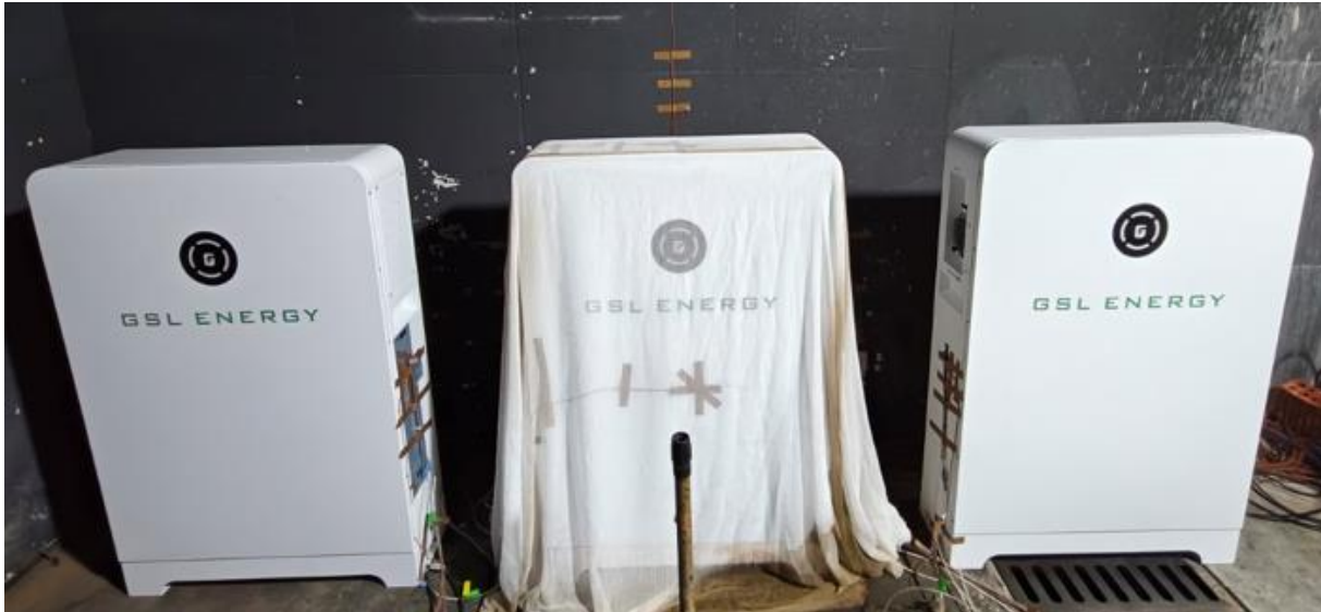
Figure 20. Photo of initiating and target BESS Units after test
